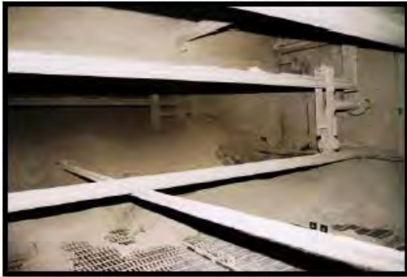
Rake Style Sootblowers
