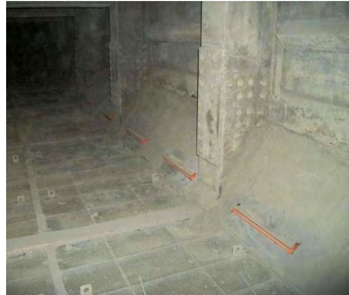
Discharge nozzle installed across front wall.
