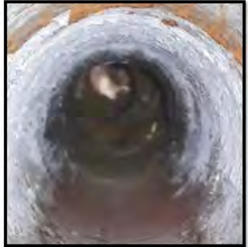
Close up view of the ID of the acoustic cleaner's bell sections.
