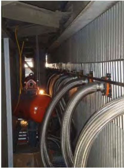
Ash Sweeper System installed on SCR
